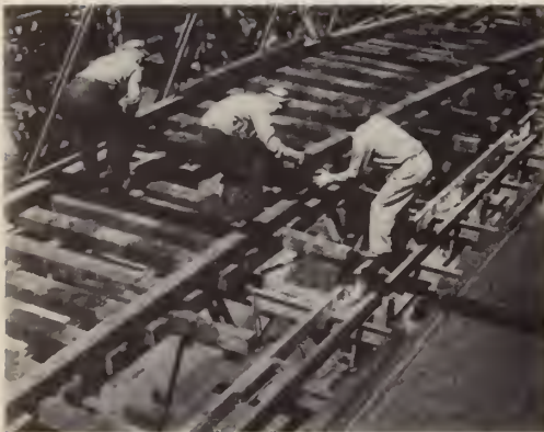
After removal of tracks, ties and guard timbers were taken out in sections.
